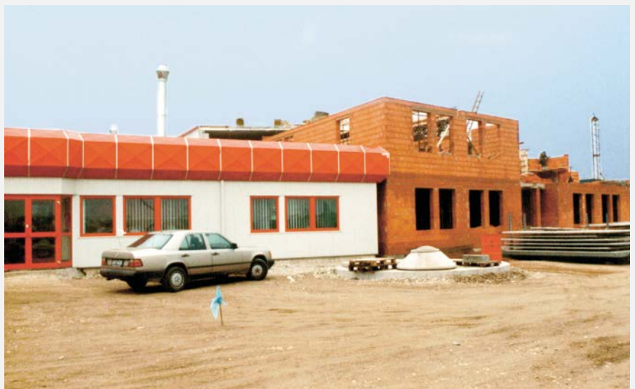
The first production facility of what was to become the POLYTEC GROUP was built in Marchtrenk, Upper Austria in 1988. Almost immediately after its completion, the location was enlarged in the course of the first business acquisition.
