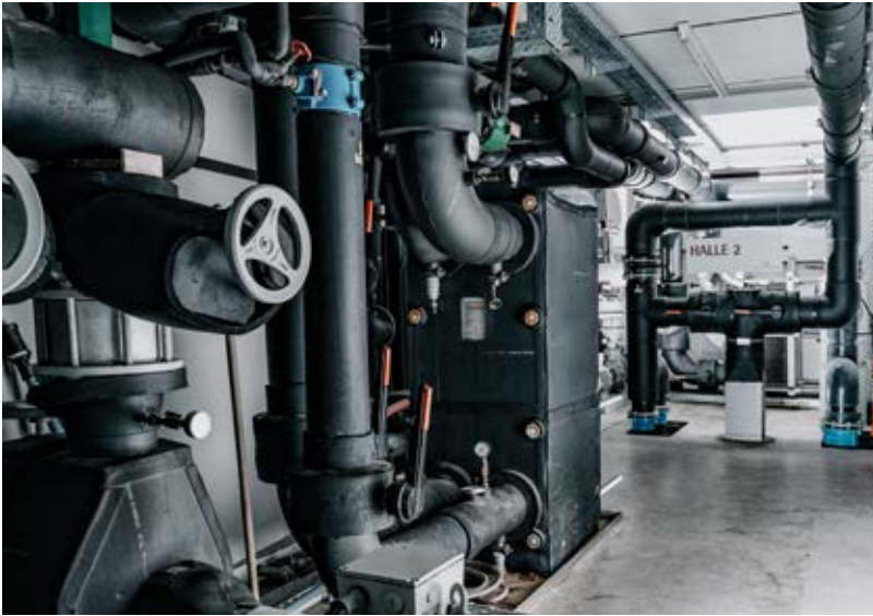
At the Ebensee plant, the injection moulding machines are cooled with groundwater.
