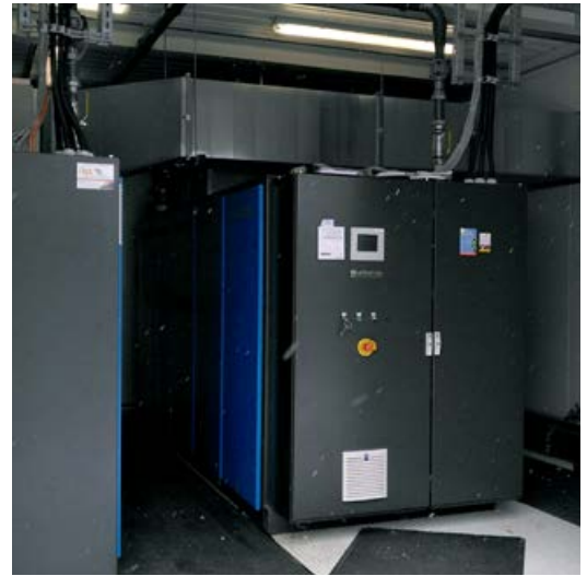
Two cogeneration modules provide the POLYTEC location in Altenstadt with a reliable, clean and favourably priced energy supply.
